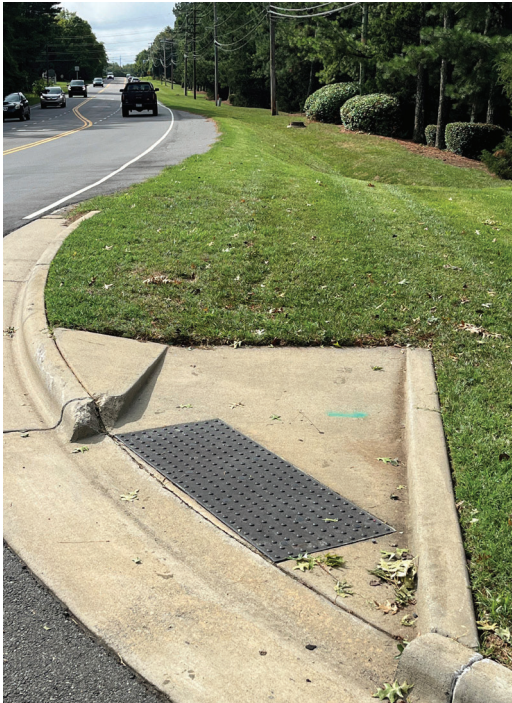
Connection point at the north end of the project at Sanel Point Drive looking south.
